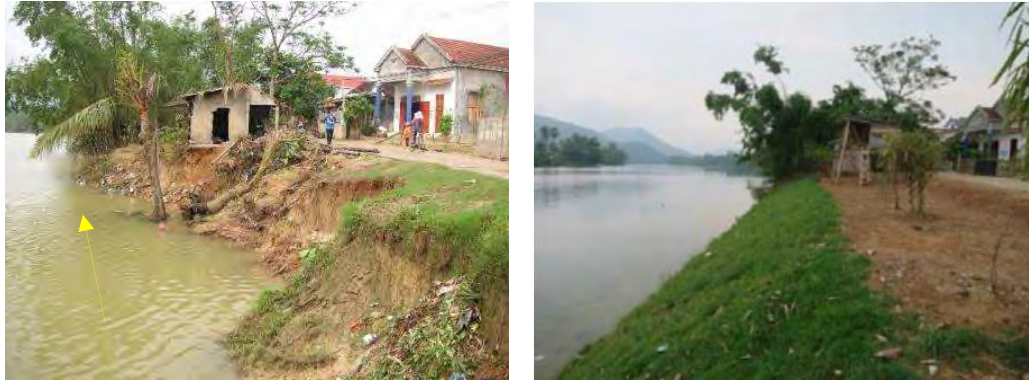
Photo 3-4-1 Before/After of construction in Quang Binh province (Series of 6 groins and slope protection)
