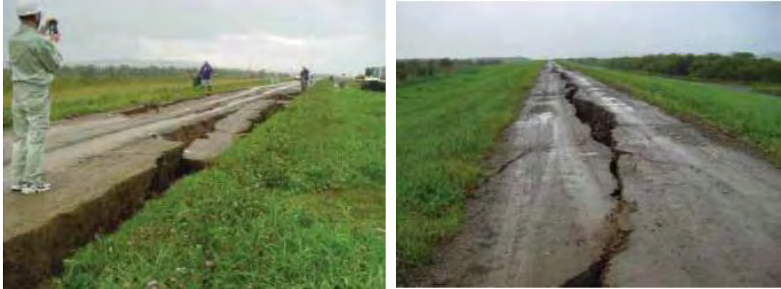
a), b) Longitudinal Crack on Dyke Crown by Earthquake
