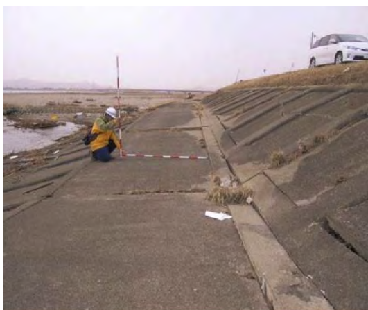
g) Caving at Berm by Tsunami and Earthquake
