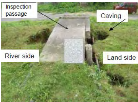
j) Caving at Drainage Culvert
