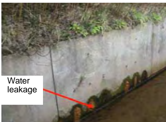
Water Leakage in Drain
