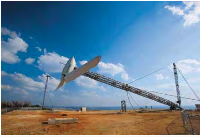
Structural reengineering of foreign-made WT tower to ensure compliance with Japanese standard
