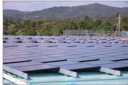
Survey, planning, and construction management of 240 kW PV project at an agricultural products processing plant in Higashi Village (Okinawa mainland)
