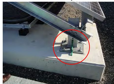
Earth wire connected to a rack
