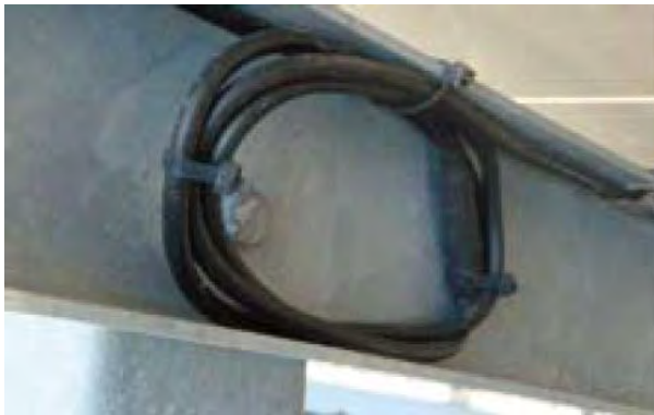
Storage of excess cable
