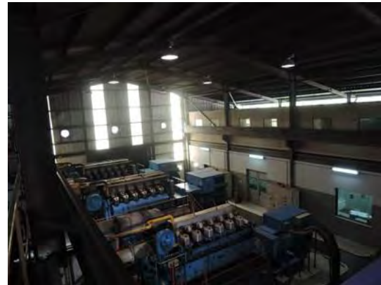
Figure 3.2.5-9 Generator room (SET 6P-8P)
