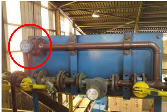
Figure 3.2.6-12 SET 8P Around the flow meter (Valve failure)
