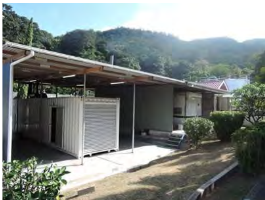
Figure 3.2.5-10 Container type generator (SET M4-M6)
