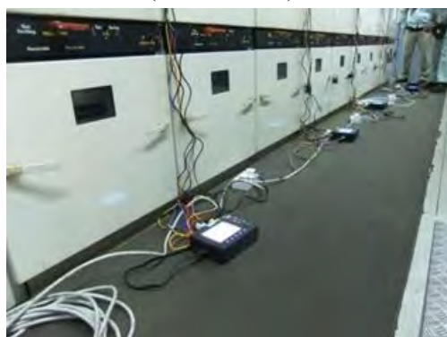
Installation of measuring instruments for load rejection (Praslin Island)
