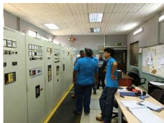
Figure 3.2.5-17 Central control room
