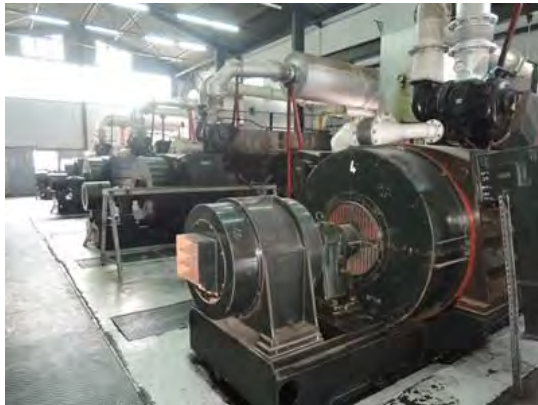
Figure 3.2.5-8 Generator room (SET 1P-4P)
