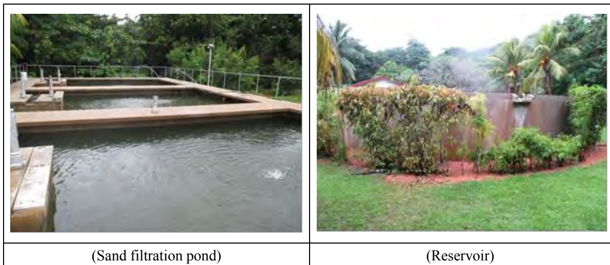
Figure 2.5.1-3 PUC owned groundwater filtration facility
