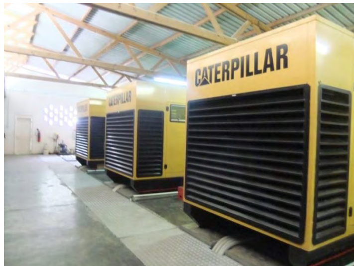
Figure 2.5.3-4 Diesel generation facility
