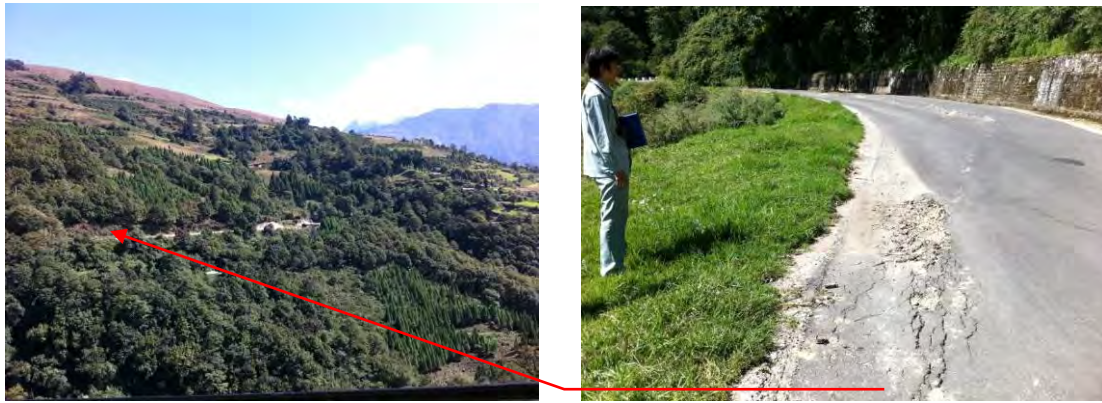
Figure 3.4.7 Deform and Cracks on the Pavement in the Landslide (Source: JET)
