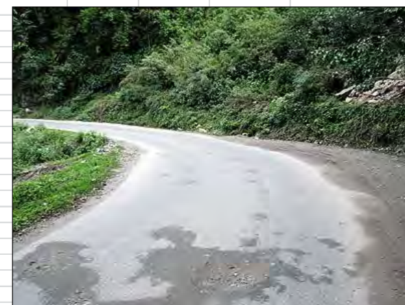
Clearance between road and the debris from end side
