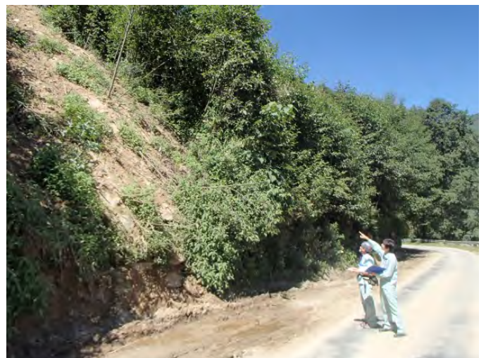
Calibration works for slope inspection by the JICA Expert Team, Trongsa, 2 October 2014
