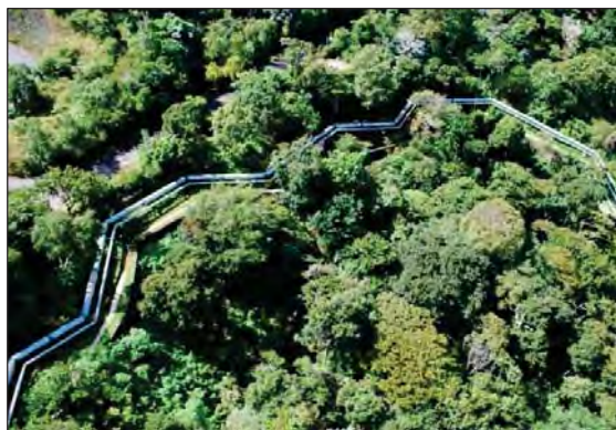
Figure 18: Pipelines at the Berlin Geothermal Project, El Salvador
