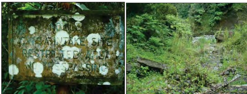
Figure 36: Destroyed CWSA intake on the Rabbaca River in the Project Area
