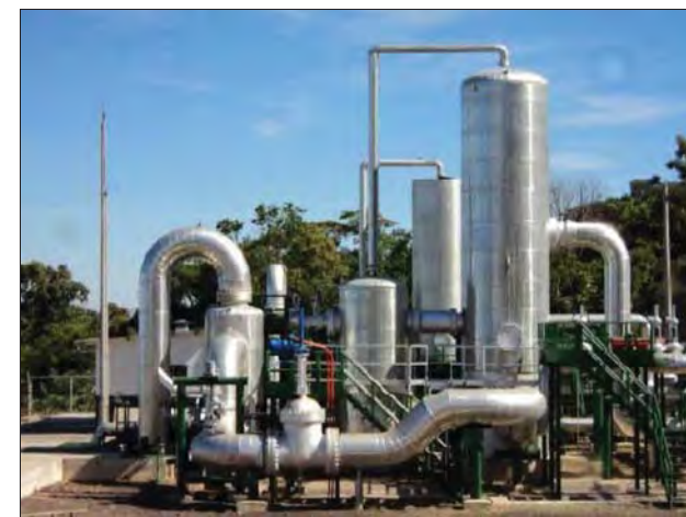
Figure 17: Separator Station at the Berlin Geothermal Project, El Salvador
