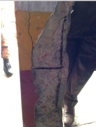
Corrosion of existing main reinforcing-bar in columns
