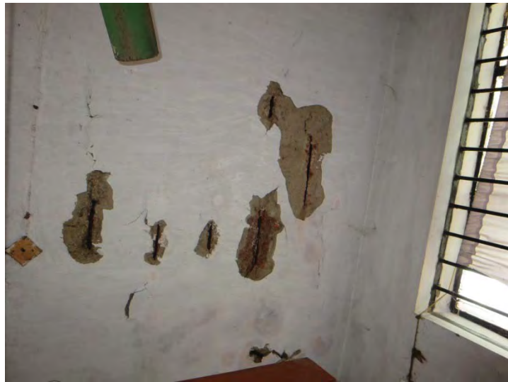
Corrosion of reinforcing-bar in existing slab
