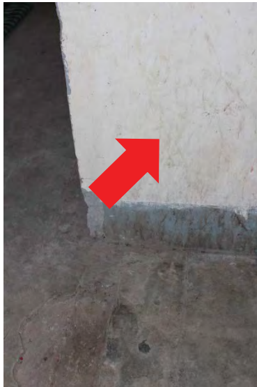
Situation of deterioration
