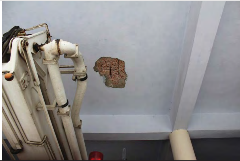
Corrosion of rebar
