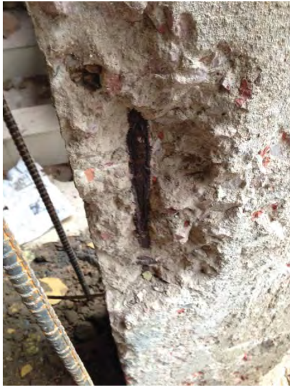
Corrosion of existing main reinforcing-bar in columns
