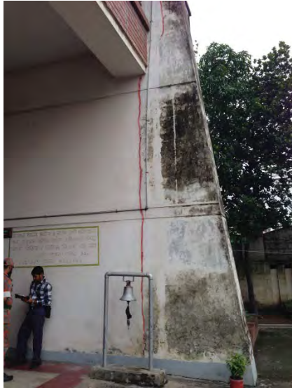
Cracking with settlement of building
