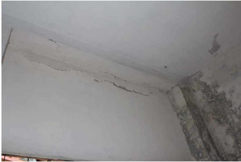
Corrosion of existing reinforcing-bar in beams
