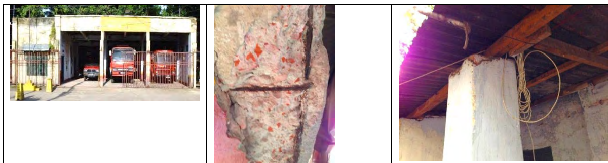
Photo: Actual states of Palashi Barak Fire Station (Built in 1947, the building has aged. The plaster has detached from the columns, and reinforcing bars are exposed and rusted. Concrete is brick chips. It is judged difficult to retrofit, and should rather be rebuilt.)
