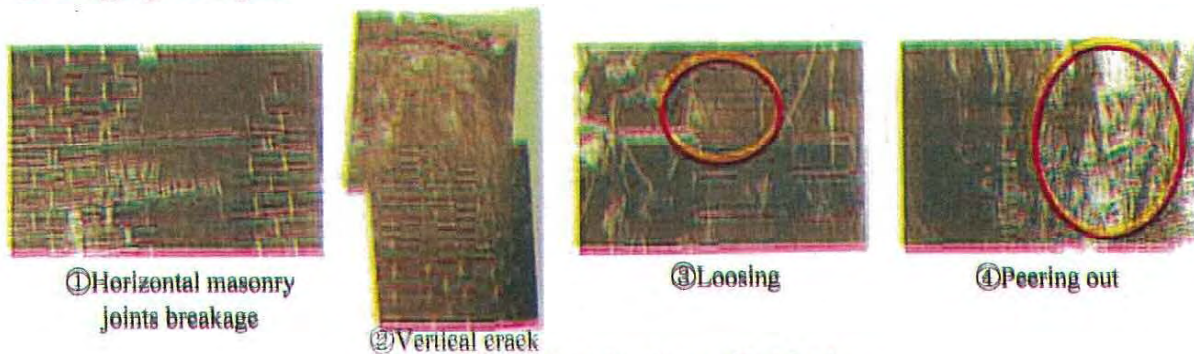
Fig4.2. Major deteriorations of brick pier
