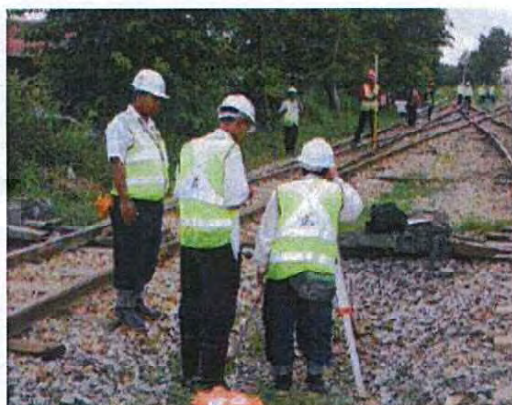
Measuring at turnout
