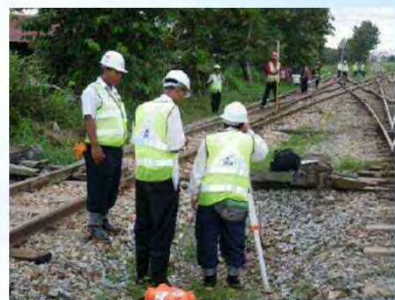
Measuring at turnout
