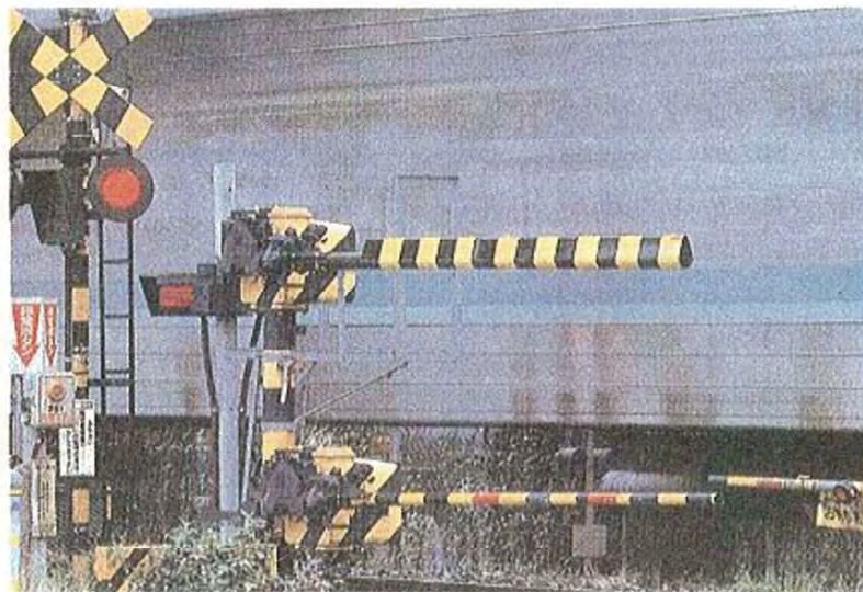
Photo 40.11 Example of large-size barrier device
