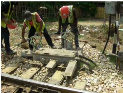
Motor Raising of turnout
