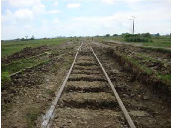
(1) Track settlement into road bed
