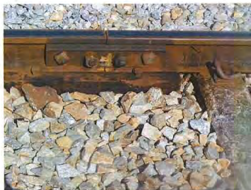
Short sleeper at joint
