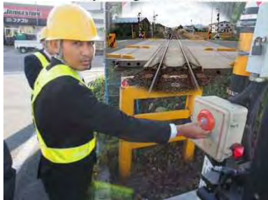
Level Crossing Emergency Call Button
