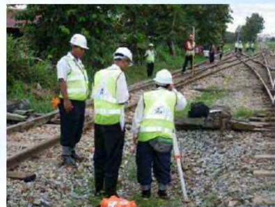
Measuring at turnout
