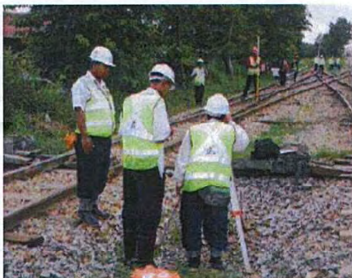
Measuring at turnout
