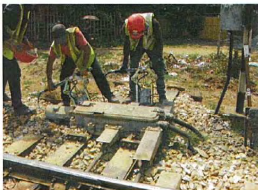
Motor Raising of turnout
