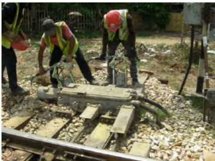
Motor Raising of turnout
