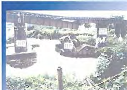
Breakage of Pier due to scouring (JR Hanawa Line in 1997)
