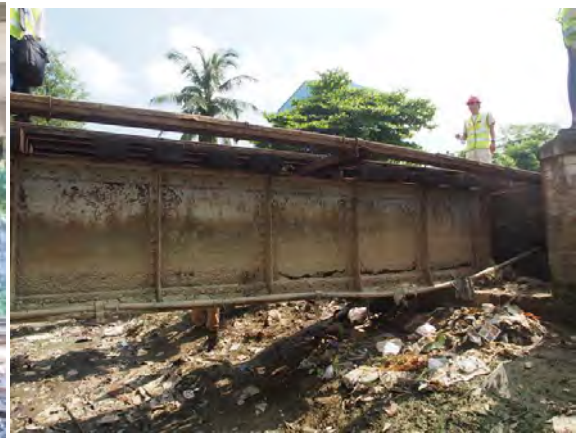
(4) No.8 Bridge 主桁腹板の孔食
