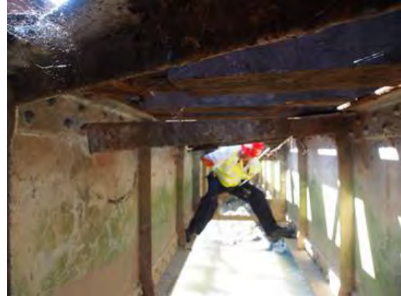
(2) No10 Bridge ラテラル脱落・横揺れ
