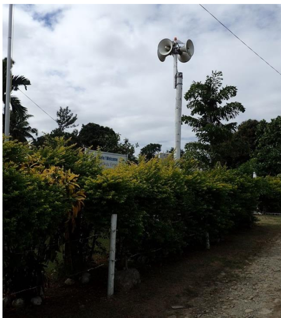
Installed siren through the IWRM project [Sikituru Village located downstream of the Nadi River]
