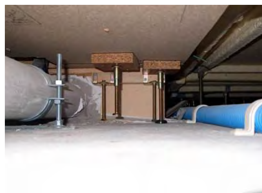
Figure 2 Piping System under Floor Panel Units
