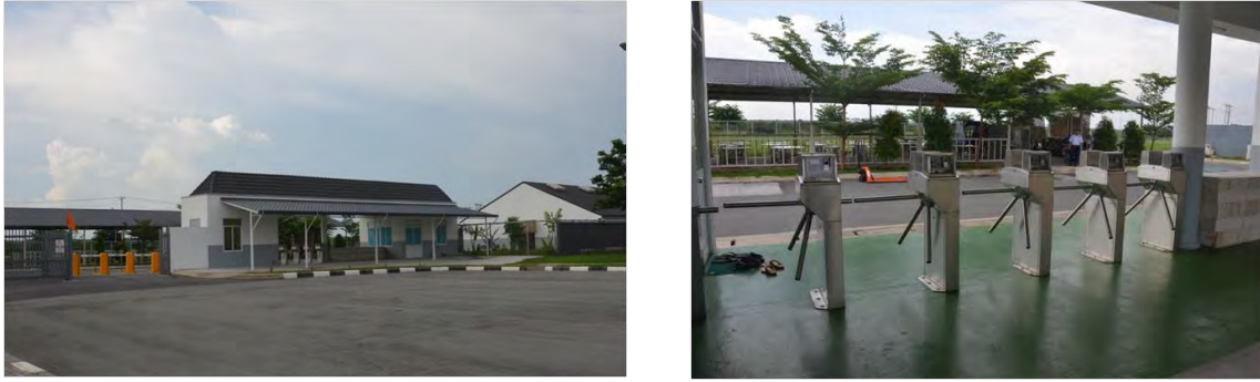
Figure 3-52 Case of Relaxing the Operational Rules by Automatic Security System (Ascendas IP)
