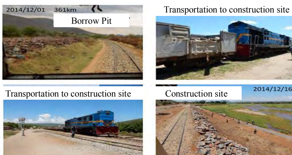
Figure 10.71: Transportation of Crushed Stone from Borrow Pit at Km 361 to Construction Site at Km 315
