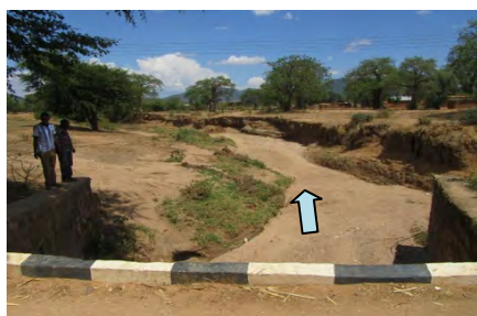
A: Sediment Deposition and Riverbank Erosion (17 Dec. 2014)
