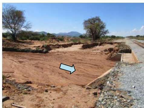
A: Condition of Remarkable Deposition (RW7)
