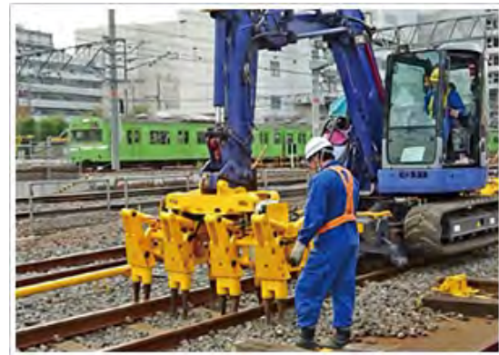
16-Tool Tie Tamper
