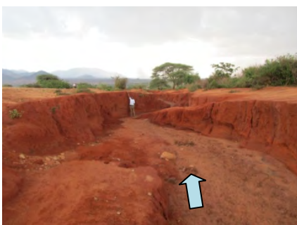
A: Eroded Road Gutter
