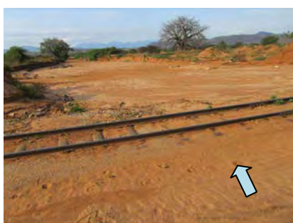
E: Obstructed the Culvert in the Current River Channel
