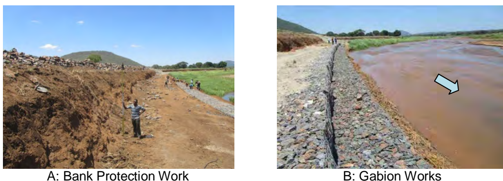
Figure 7.25: Condition of Site Km 315.1
