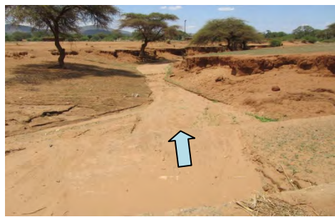
D: Condition of Riverbank Erosion at Downstream Side
