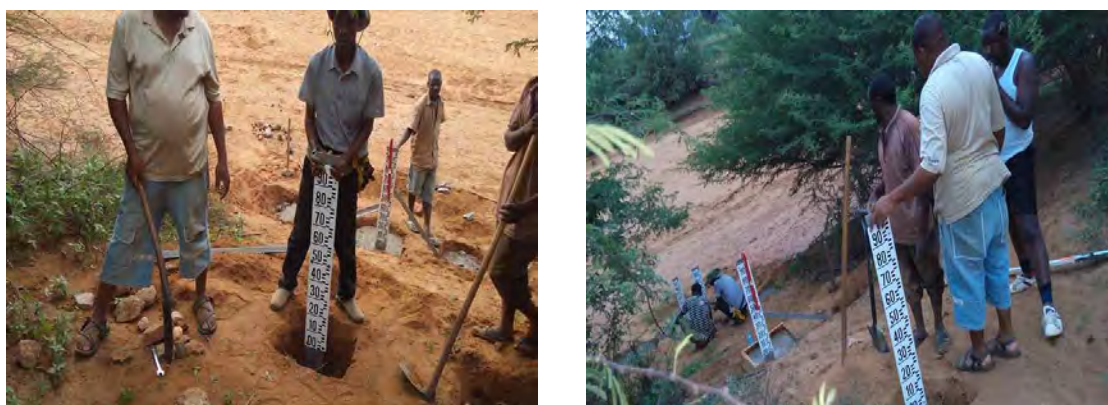
Figure P.5: Construction of the Water Level Gauges in the Mzase River at Gulwe
