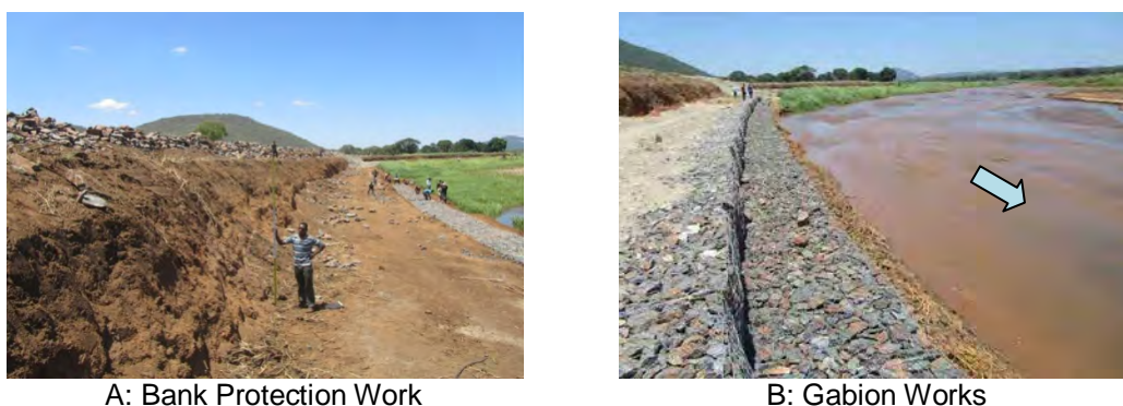
Figure 7.25: Condition of Site Km 315.1
