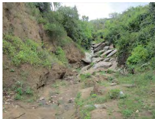
Unnatural Contact with Slope
