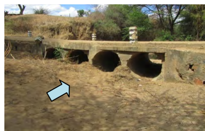
B: Little Sediment Deposition
