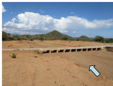
B: Risky Bridge against Flood
