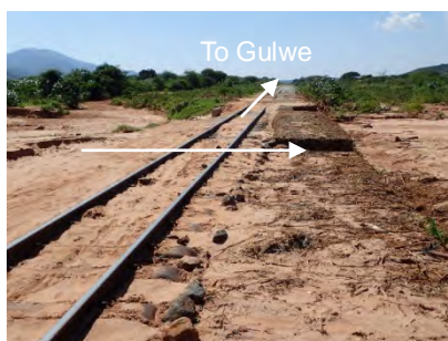
Figure 5.17: Near CL 349.8B (buried)
