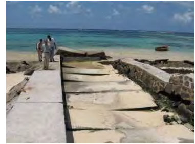
Photo 5-2-21: Outlet B Structural Damage by Erosion (April 2011)
