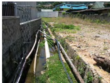
Photo 5-2-2: Obstacle in River Maintry
