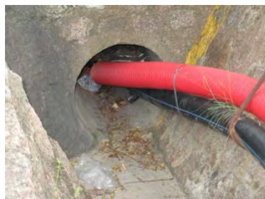
Photo 5-2-5: Obstacle near junction of 5th June Ave. and Manglier Rd.
