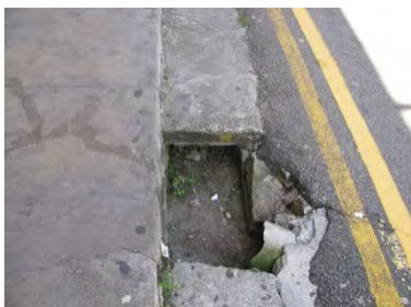
Photo 5-2-4: Present side drain at Market Street
