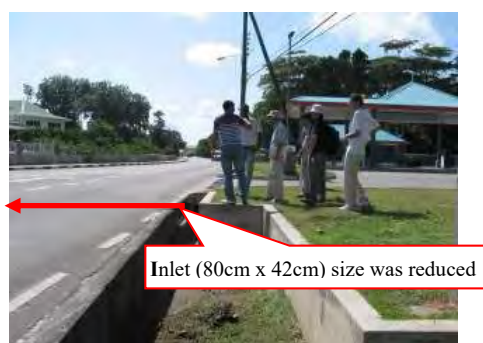
Photo 5-2-15: Narrow drainage inlet (A) (April 2011)
