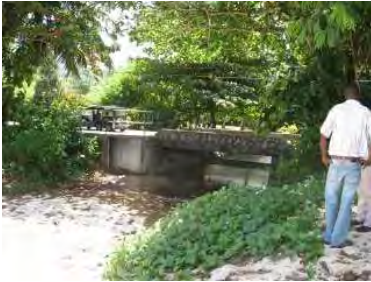
Photo 5-2-19: Outlet A river mouth clogged (April 2011)
