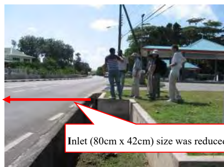
Photo 5-2-6: Narrowed drainage inlet (A) (April 2011)
