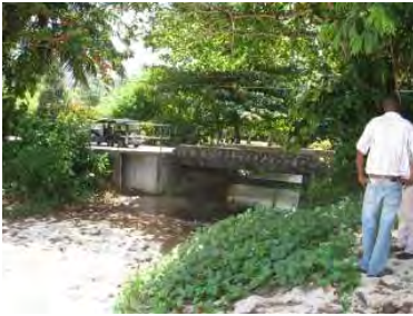
Photo 5-2-10: Outlet A river mouth clogged (April 2011)
