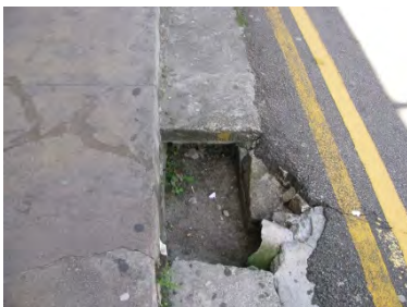
Photo 5-2-4: Settled side drain at Market Street
