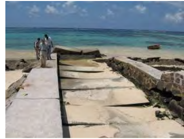
Photo 5-2-12: Outlet B Structural Damage by Erosion (April 2011)
