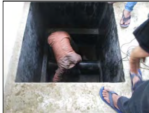
Photo Title Device Operation Training Description Fixing sensors on PVC pipe Venue CWASA Training Center Date Taken 2016/Jan/01 (Fri)
