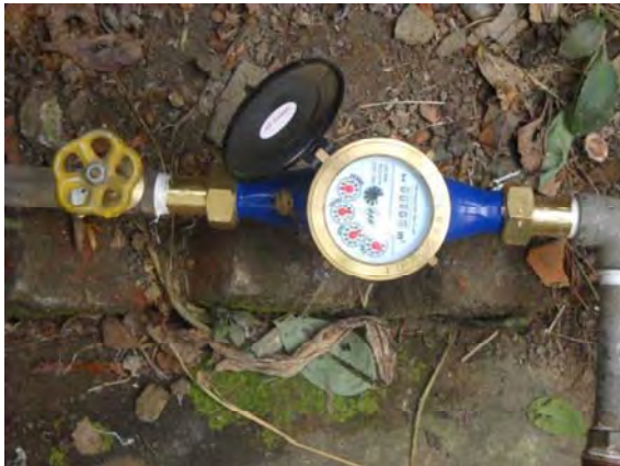
Photo 4.1 Installed water meter
