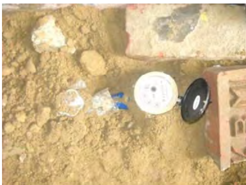
Photo 4.10 Low Position of Water Meter
