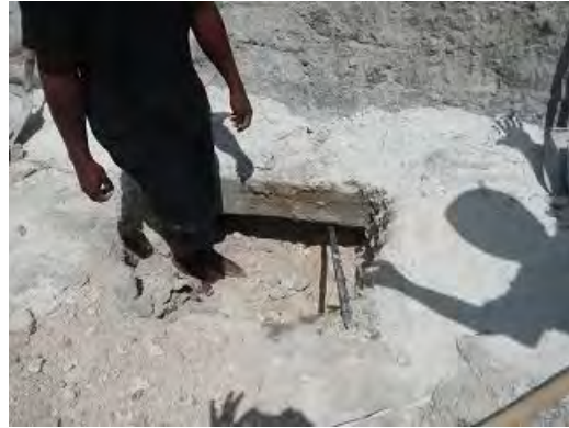
Large cavity under seawall
