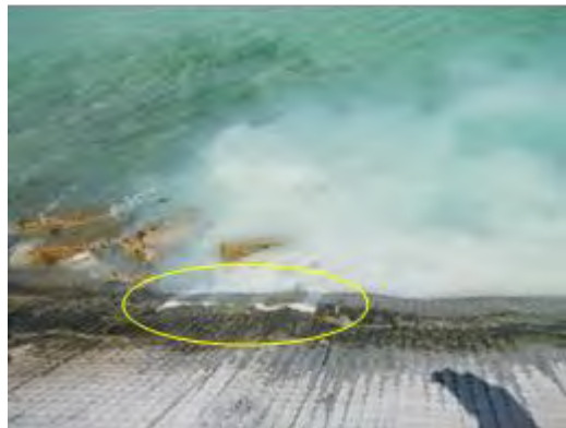
Outflow of filling materials from cracks
