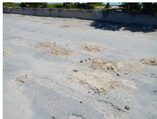
Natural compaction by vehicles
