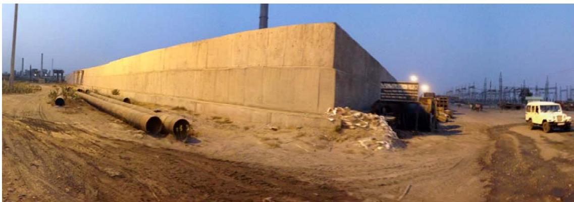
Survey of conditions at Units No. 6/7 (Units No.6/7 ash handling system, cooling tower)
