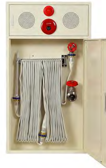
Fire Hydrant Box Located in Station Area
