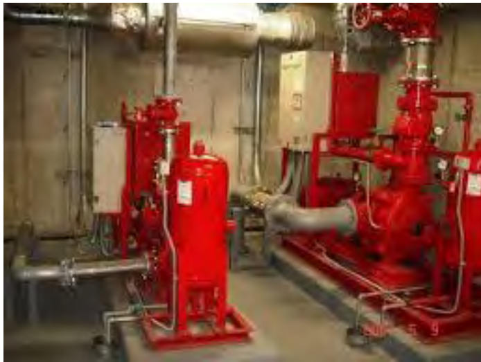
Fire Hydrant Pump Located B4 Fire Pump Room
