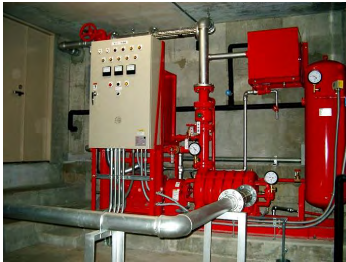
Sprinkler Pump Located B4 Fire Pump Room
