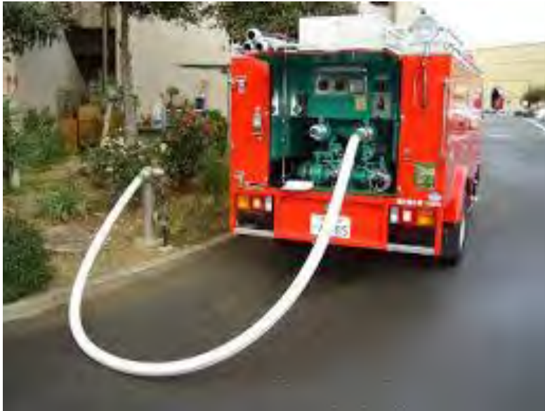
Fire Engine Supply water to Siamese Connection
