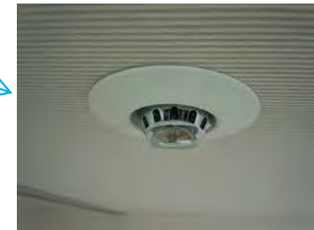
Sprinkler Head for false ceiling
