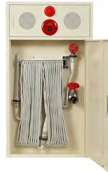
Fire Hydrant Box Located in Station Area
