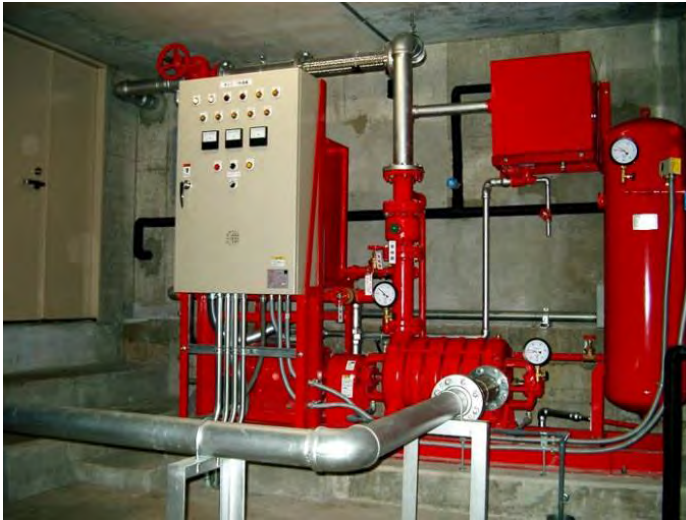
Sprinkler Pump Located B4 Fire Pump Room
