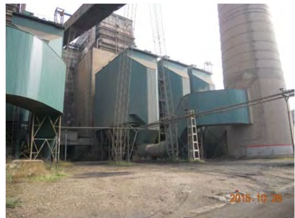
Photo 3-12b 3 ESP lines installed for each boiler (shown here: A-3)
