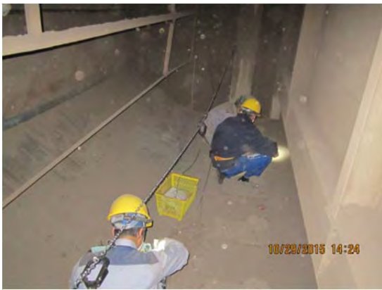
Photo 4-2a View of inlet side measurement
