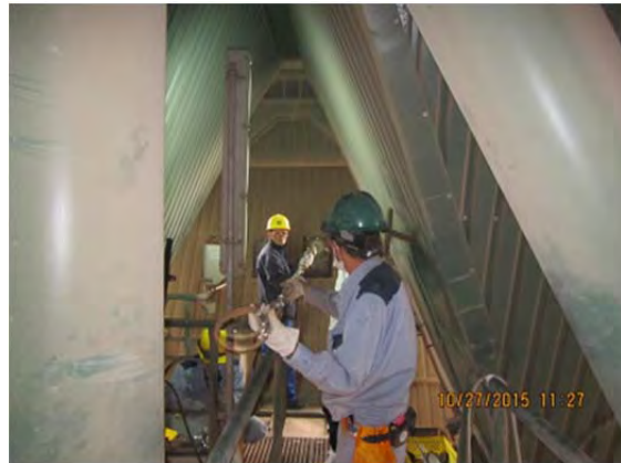
Photo 4-2b View of outlet side measurement
