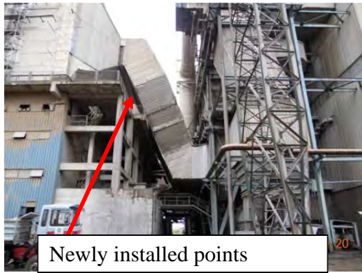
Photo 4-4a Measurement point at inlet of ESP
