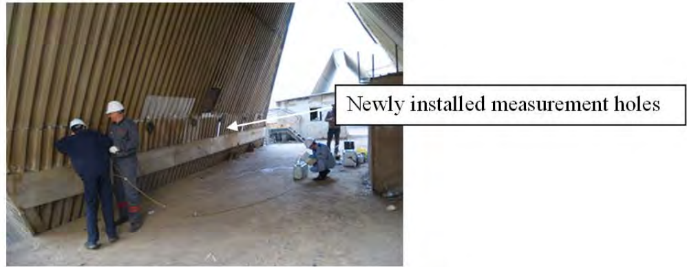
Photo 4-5a View of dust measurement at inlet of ESP
