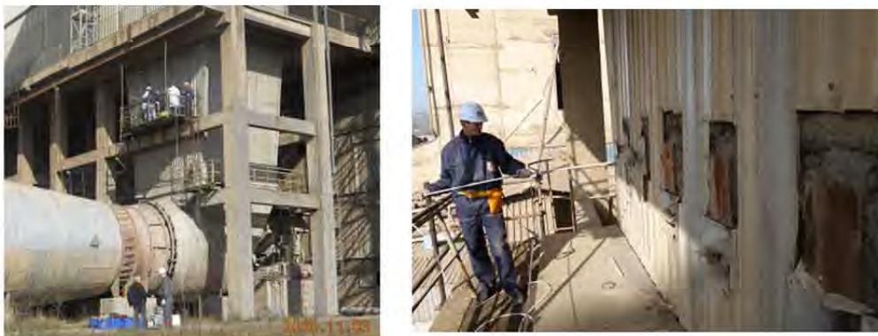
Photo 4-5b View of dust measurement at outlet of ESP
