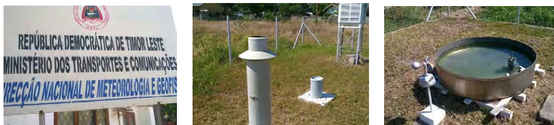
Figure 1-2-1 Meteorological Observation Equipments in President Nicolau Lobato International Airport
