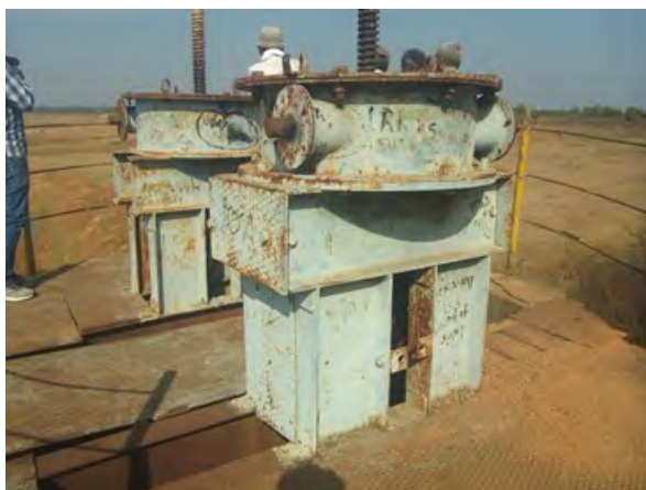
Malfunctioned old intake gates shall be replaced with new ones. (West Godavari District)
