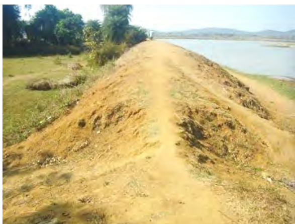
Tank bund is seriously damaged, which shall be improved along with intake structures, spillway and canals. (Vizianagaram District)
