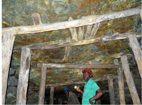
8 : State of roof rock near gallery inlet
