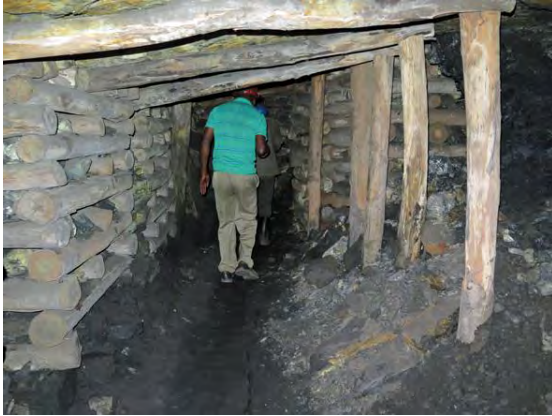
7 : State of supports near gallery inlet
