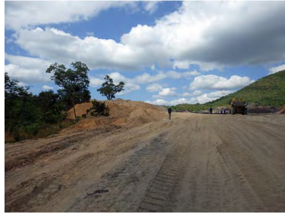
2 : State of road
