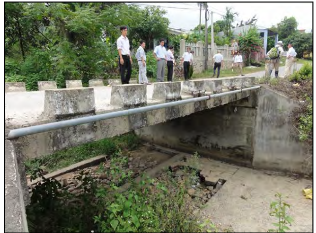
Photo 5.20 Side stream in Section d-e. Pipe crosses under the stream right to left.
