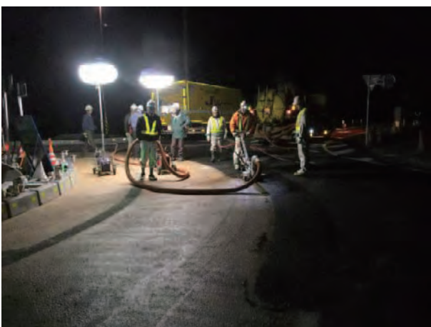
Flood lights for work area
