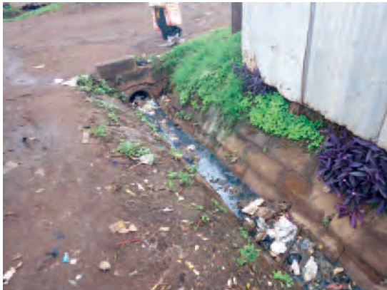
Silted drainage on unmaintained road
