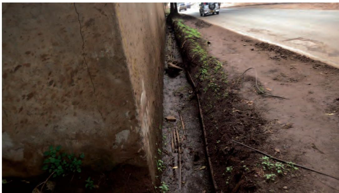
Example: Illegal pipes are found after cleaning the ditch during the Initial Mobilization Period
