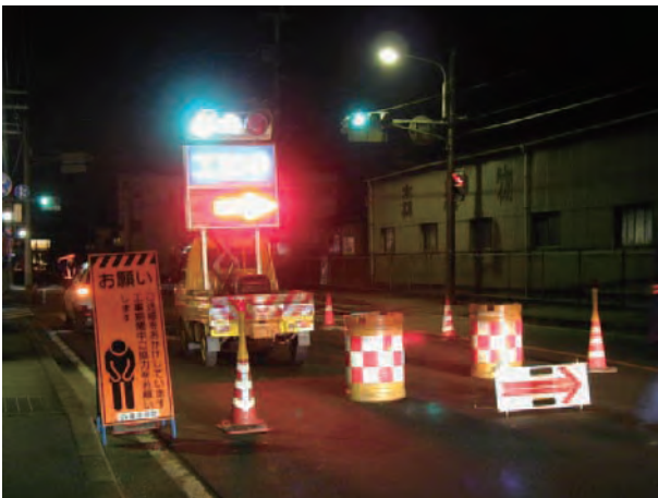
Luminous arrow board on truck and cushions
