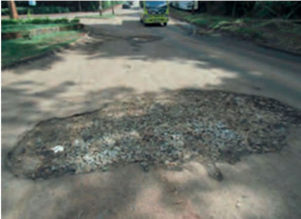
Potholes left unattended
