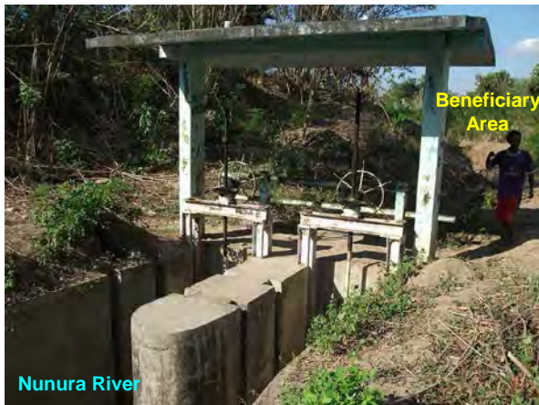
Intake facility from Nunura River
