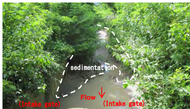
Picture : Situation of sedimentation in front of intake-gate (Feb. 2014)
