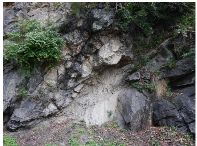
Photo 5-18 A crushed dip-slope crack on the left bank along the main road
