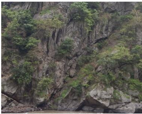
Photo 5-17 Enlarged above dip-slope crack on the right abutment, where some parts are crushed
