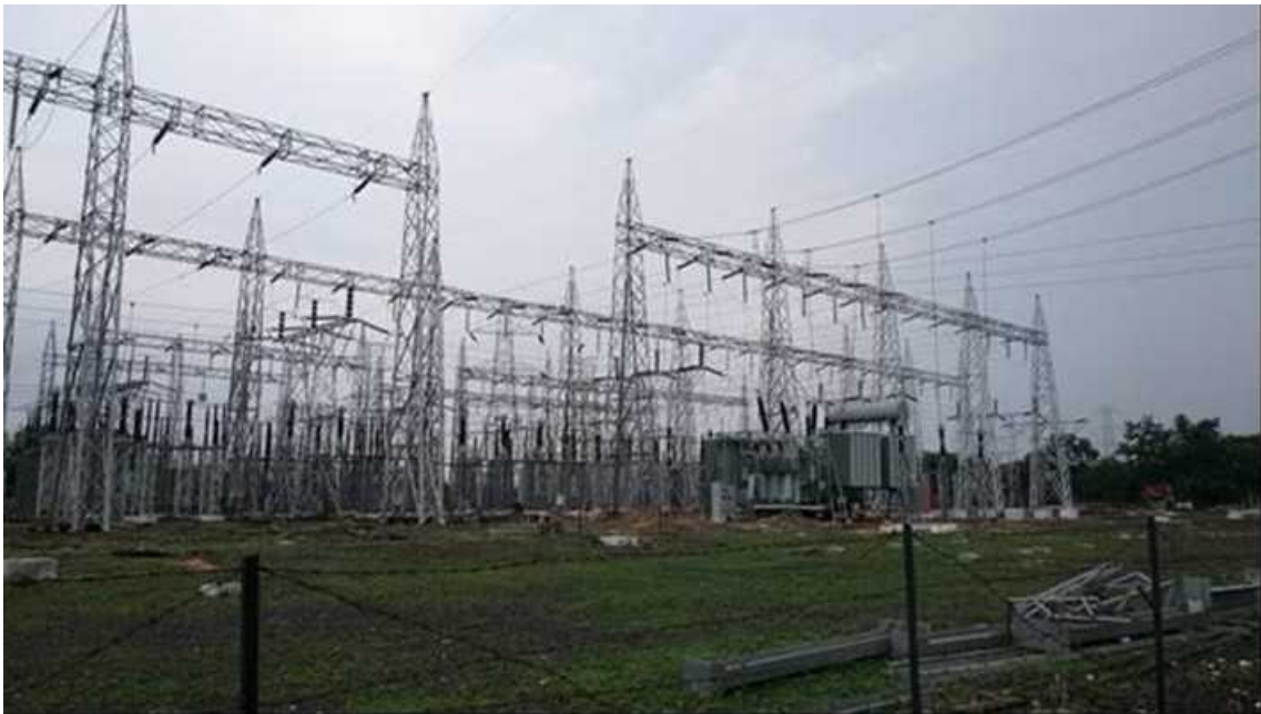
Figure 2-16 220kV Feeder Bay (Jabalpur 220kV Substation)
