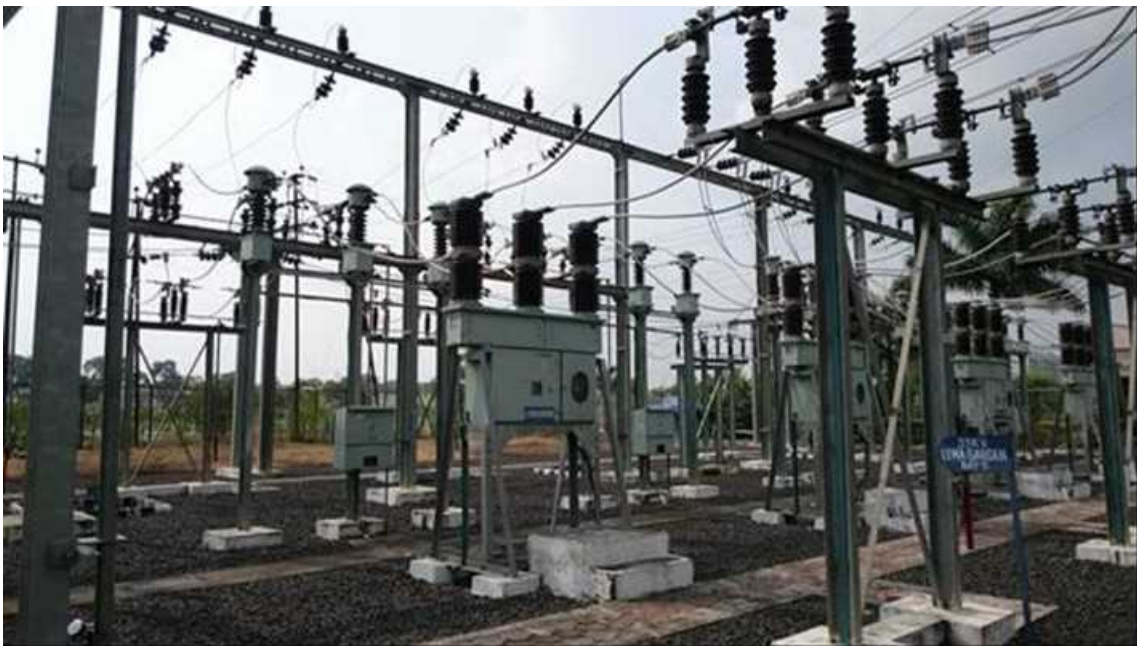
Figure 2-18 33kV Feeder Bay (Marhotal 132kV Substation)
