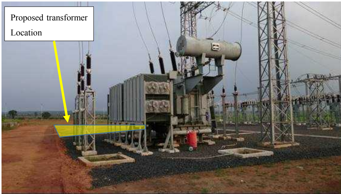
Figure 2-33 Transformer Installation Location on Tejgarh S/S
