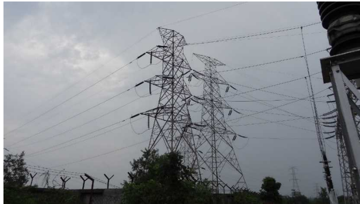
Figure 2-6 220kV Transmission Line (Incoming Tower to the Jabalpur S/S)
