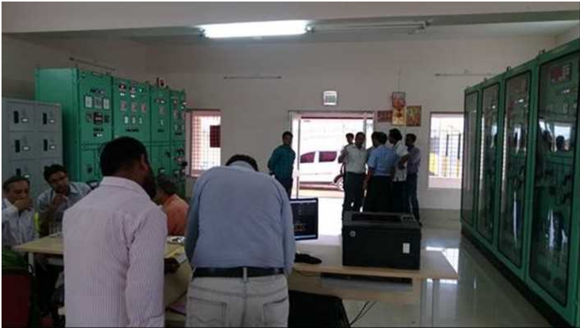
Figure 2-21 Control Panel (Tejgarh 132kV Substation)
