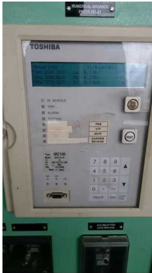
Figure 2-23 220kV Transmission Line Protection Relay Unit by Toshiba (Jabalpur 220kV Substation)
