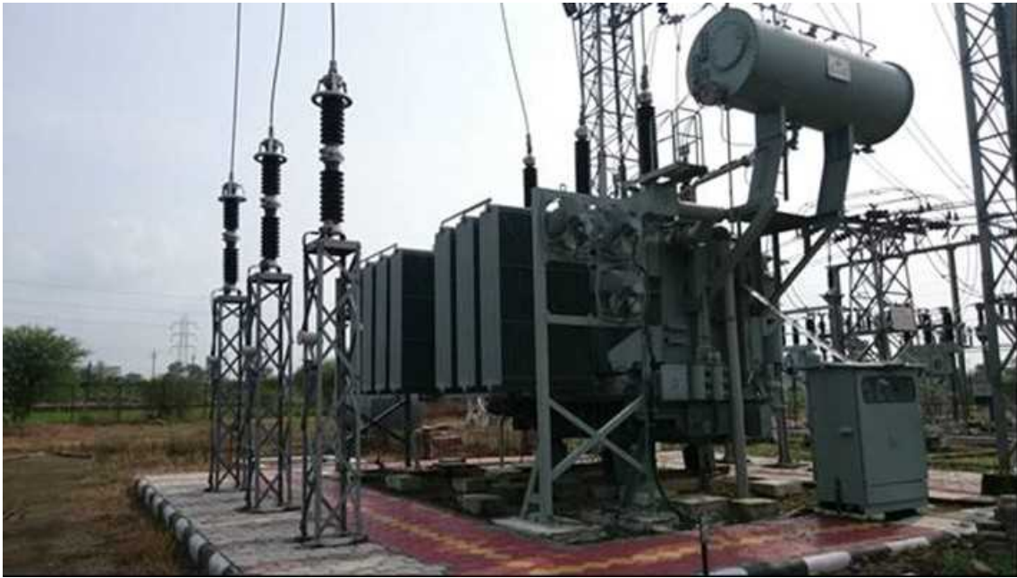
Figure 2-15 132/33kV, 63MVA, 3-phase Transformer (Marhotel 132kV Substation)
