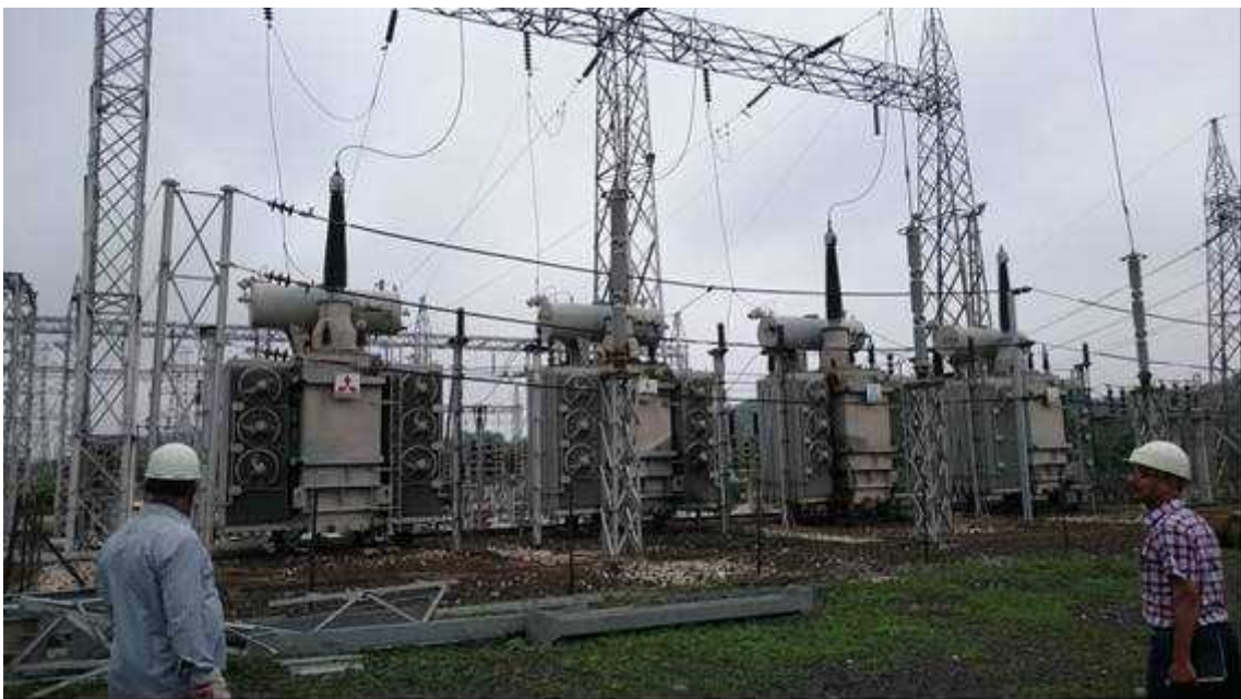
Figure 2-14 220/132kV, 40MVA x 3, Single-phase Transformer (Jabalpur 220kV Substation)
