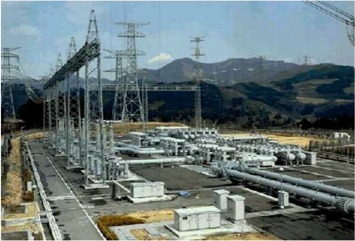
Figure 2-24 500kV Outdoor GIS Substation (TEPCO)
