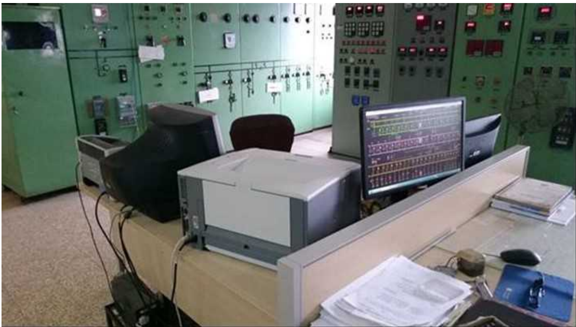
Figure 2-22 Substation SCADA System (Jabalpur 220kV Substation)
