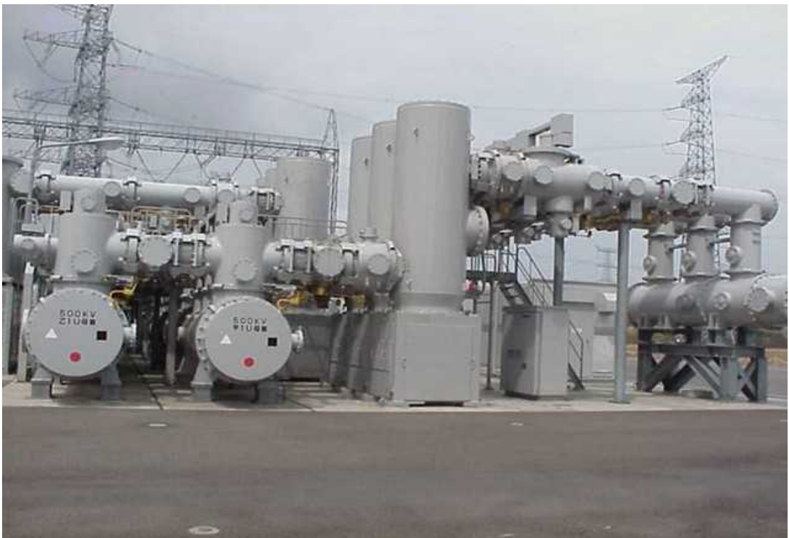
Figure 2-25 500kV Outdoor GIS Substation (TEPCO)
