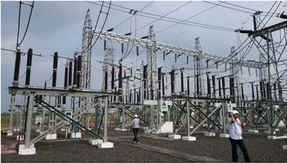
Figure 2-17 132kV Feeder Bay (Marhotal 132kV Substation)
