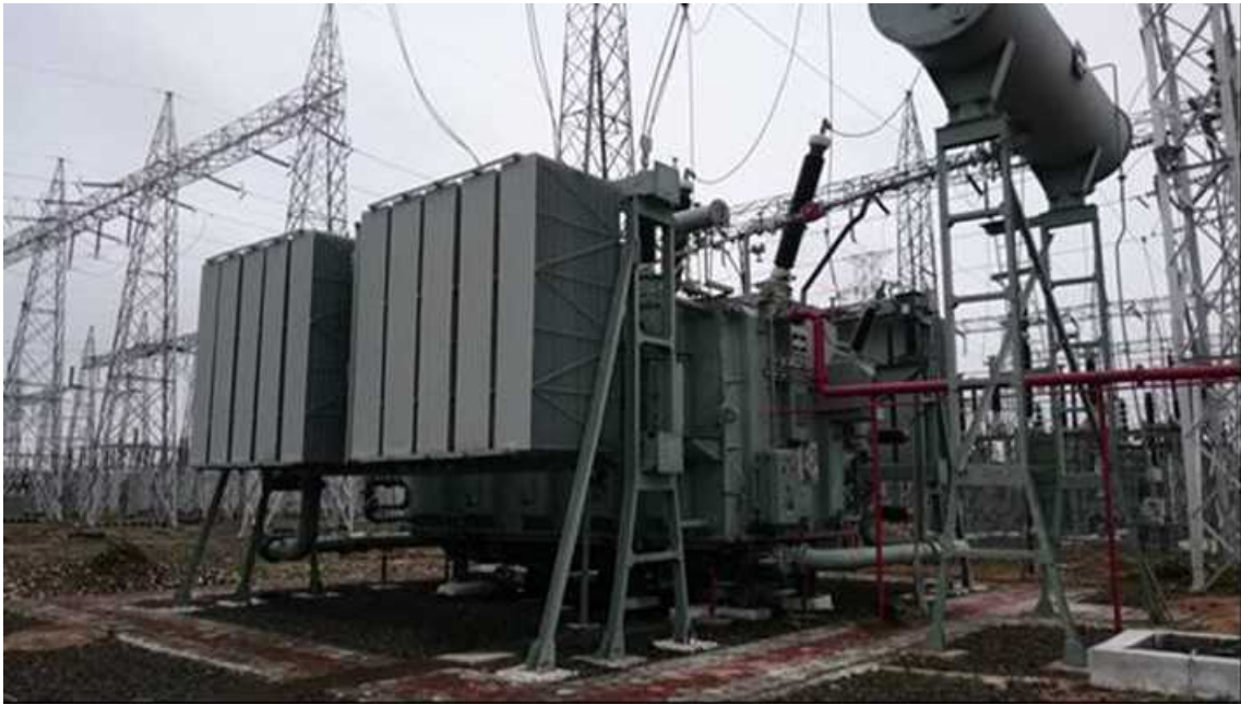
Figure 2-13 220/132kV, 160MVA, 3-phase Transformer (Jabalpur 220kV Substation)
