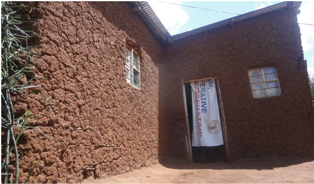
Figure 4: Second building in Bumbogo Sector affected.
