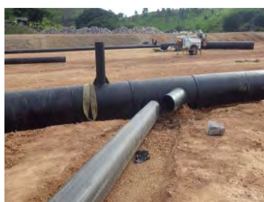
Leachate Collection Pipes (December, 2015)
