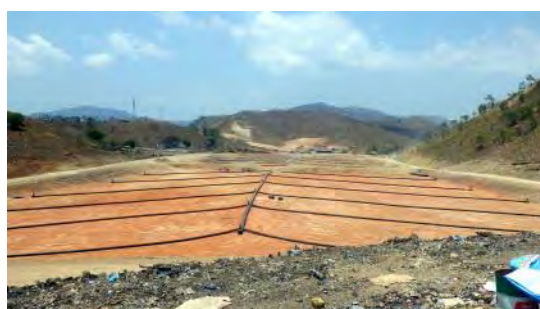
Pipe network in Cell 2 laid without preparing trenches as per the design
