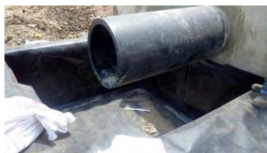
Main leachate pipe flowing into silt trap
