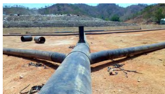
Cell 2: Branch pipes inclined upwards at junctions with main pipes
