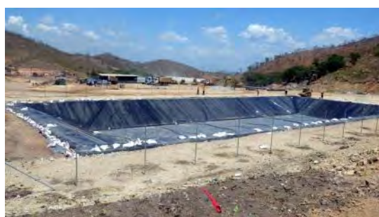
Leachate pond with HDPE and fence
