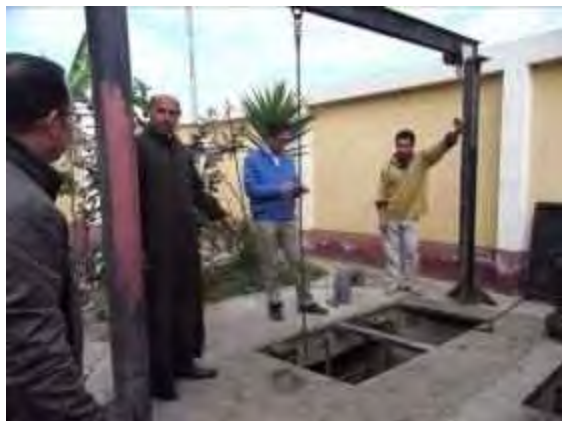
Pump facility for the sewage treatment plant in Koleaah village
