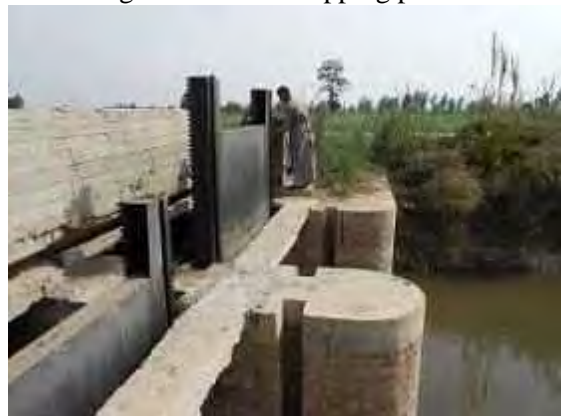
Check Gate on Shaba Canal (KM2.5)
