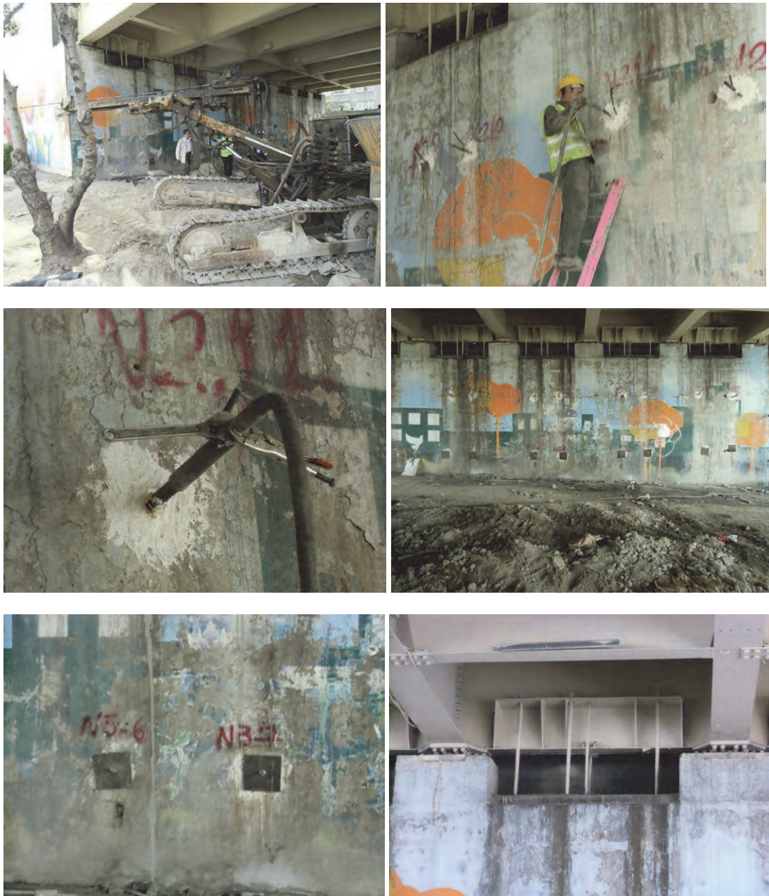
Figure 2.2.27 Photos of construction situation, Anchor installed situation, Retrofitting situation at the bearing
