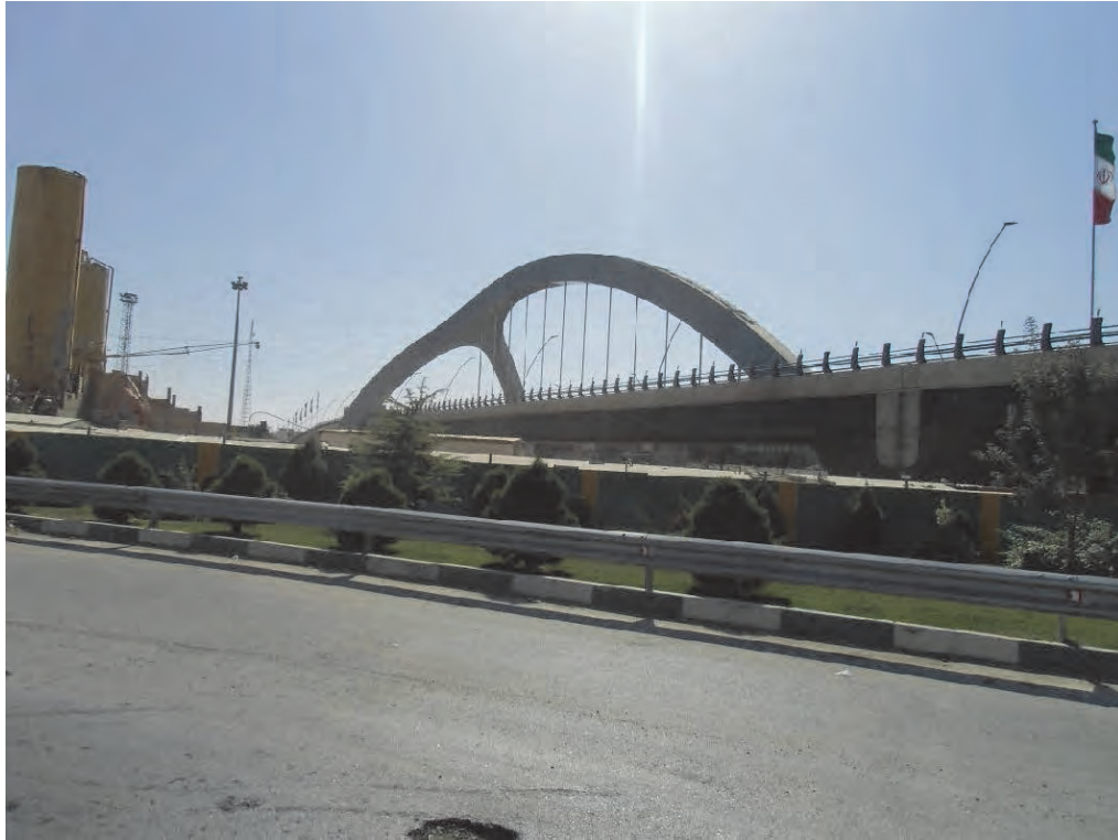
Figure 2.2.30 The bridge with an isolation damper installed at the girder end
