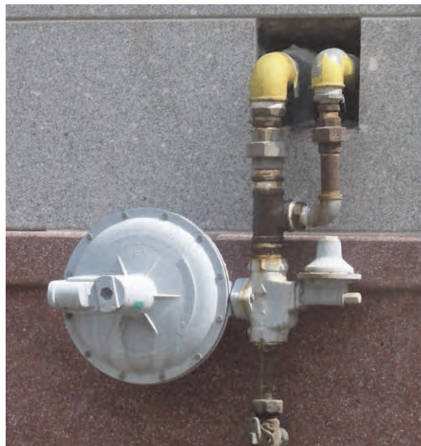
Figure 2.2.18 Regulator for pressure control attached to a house
