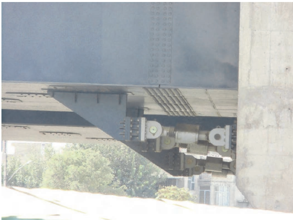
Figure 2.2.31 The isolation damper at the girder end
