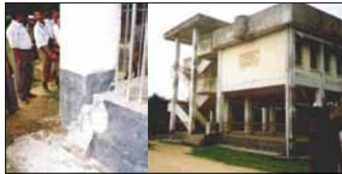
Column damaged by 1999 earthquake in Moheshkhali
